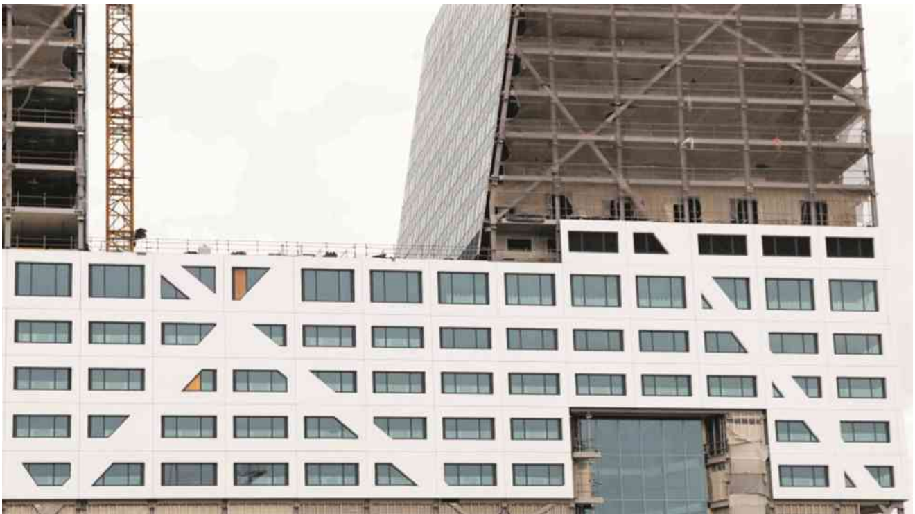
Figure 58: Installation of exterior wall panels in the construction of the Utrecht city council offices.
