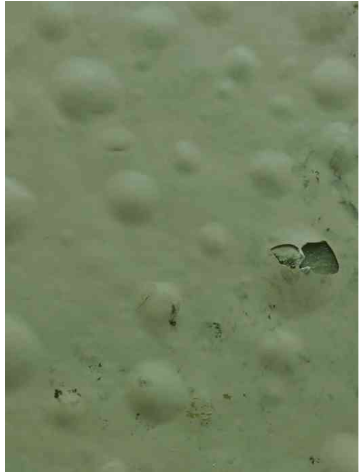
Figure 30: Damage through osmosis and hydrolysis: blistering (source: RWS-GPO)
